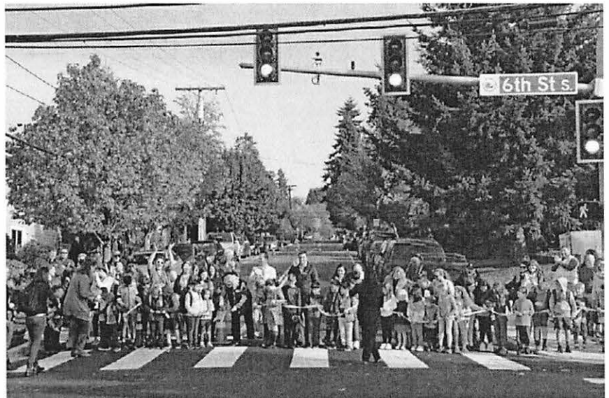
Figure 34. Sixth Street improvements, which included water, sewer, storm, sidewalk, overlay and reconstruction and traffic signals (City of Kirkland).
