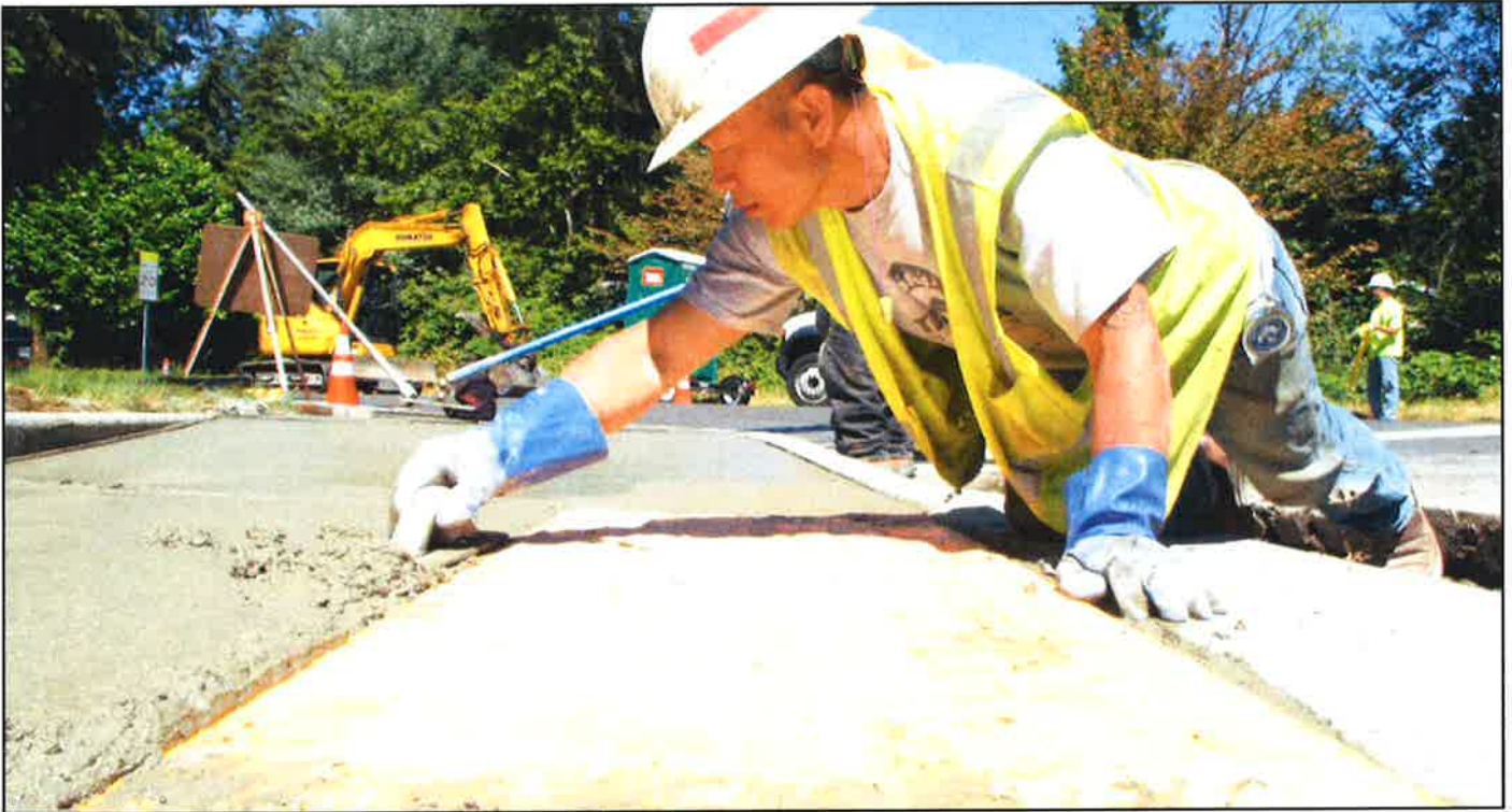
A contracted worker sculpts the concrete around the edges of a tactile warning strip along 100th Avenue Northeast, north of Northeast 125th Street. These tactile warning strips tell the vision-impaired they are about to enter a traffic zone.
